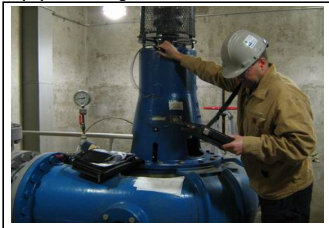
Raw Sewage Pump 1
