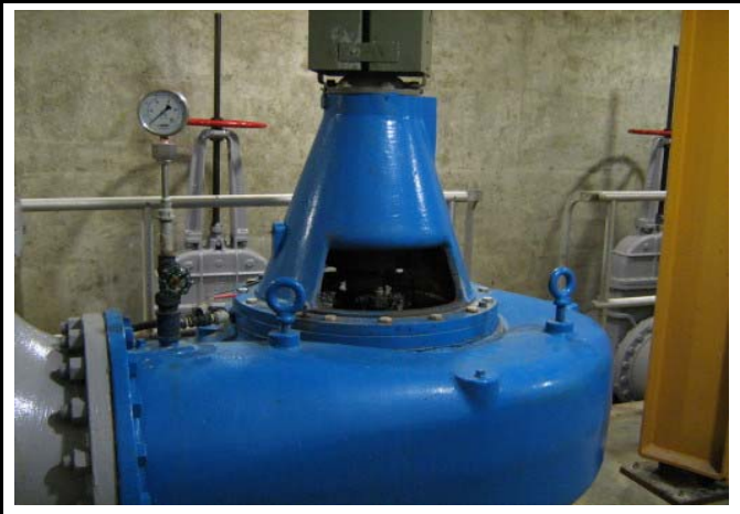
Raw Sewage Pump 3
