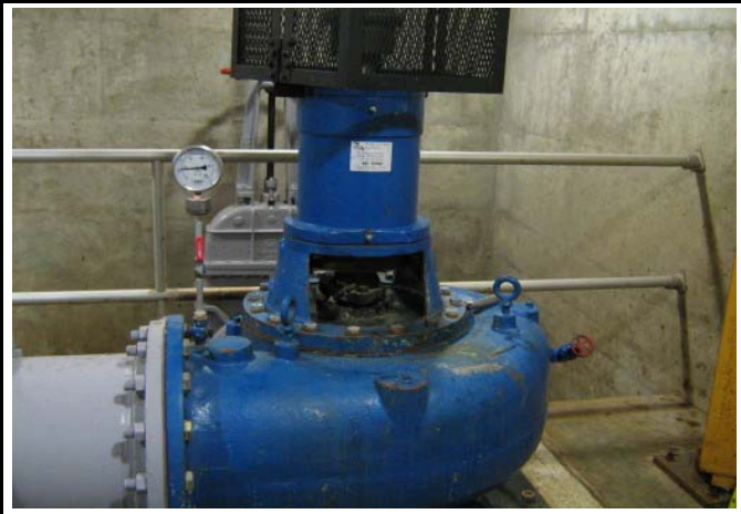
Raw Sewage Pump 4
