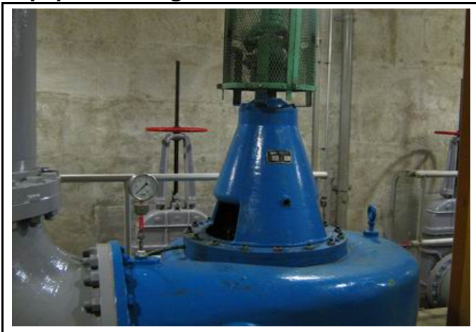
Raw Sewage Pump Diesel
